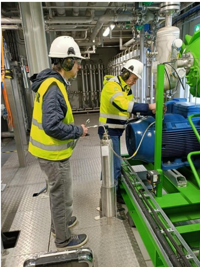
Filling of the cylinders with biomethane at the Nordsol bio-LNG installation by Jerom van Roosmalen, CEO of Nordsol.
